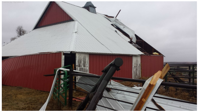
Figure 3. Photo of the tornado damage in Furnas County on November 16, 2015. The tornado was estimated as an EF-1 with winds up to 95 mph. Photo from the National Weather Service in Hastings Storm Survey Team— http://www.weather.gov/gid/nov16172015
